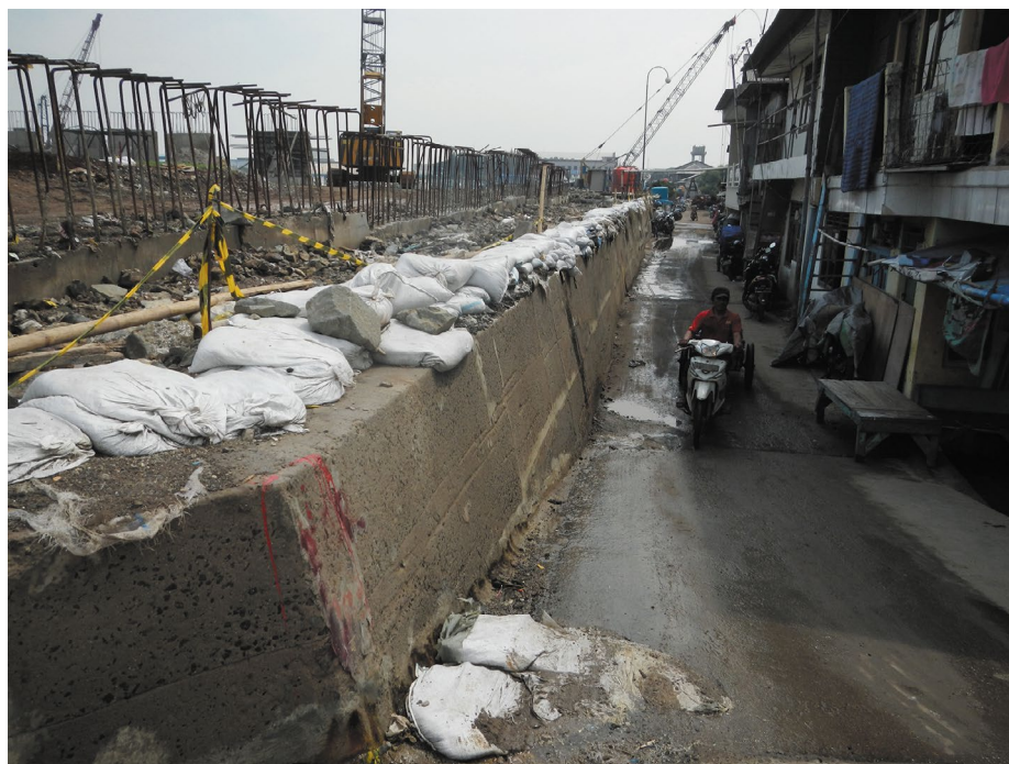
Fig. 1 | Strengthening protection of subsiding coastal areas in Jakarta. The northern part of Jakarta experiences frequent overflows of sea water over seawalls during the spring tide, which deteriorates the living conditions of residents. Seawalls were raised repeatedly as land subsidence proceeded. Photograph reproduced with permission from Japan International Cooperation Agency (JICA).
